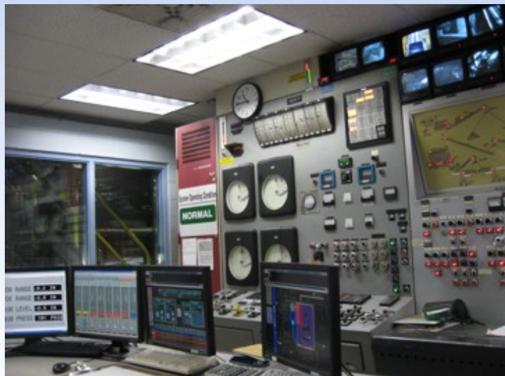
(top to down) The front of the wood burning boilers. The wood is dumped onto a moving grate where it is then burned. Two of the three boilers can burn wood. / The rear side of the wood burning boilers. / The control room at Bay Front allows for the continued observation of all activities going on in the plant.
